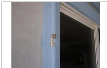
various areas with minor damage at stucco trim (EIFS)
