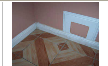
possible previous leak
