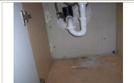
moisture stains under various bathroom sinks
