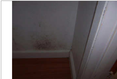
mold like substance noted in bedroom closet
