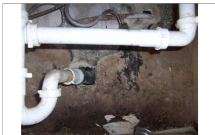
excessive mold like substance below sink.....
