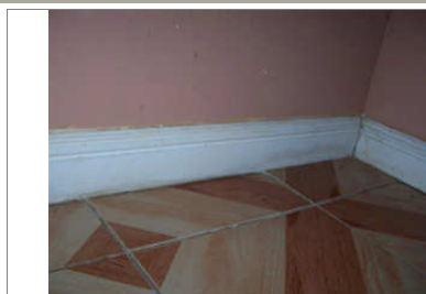
moisture stains noted
