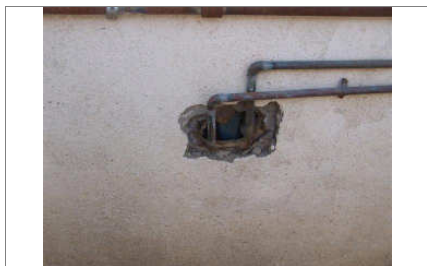
various openings around plumbing penetrations need repair/sealed
