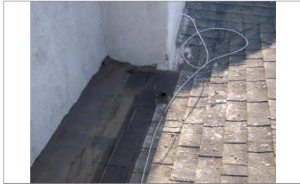
improper step flashing at roof to deck
