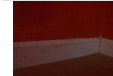
mold like substance at baseboard and at wall nearby
