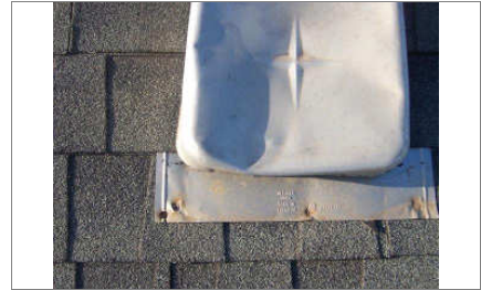
various flashing with exposed fasteners. Maintenance recommended
