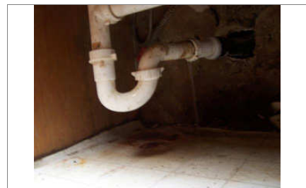
active leak at drain
