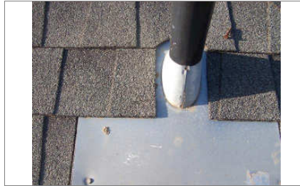
typical maintenance and seal needed at roof jack sleeves
