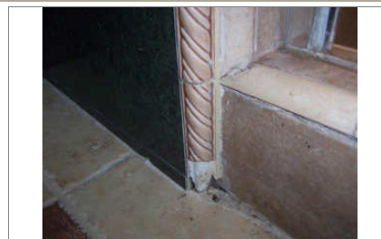
missing trim tile at shower stem wall. Recommend patching for water tightness
