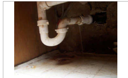
active leak at drain
