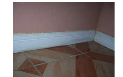
moisture stains noted
