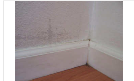
possible mold like substance appears to have been previously painted over
