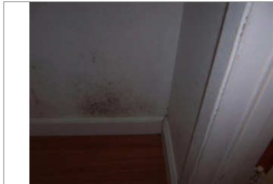
mold like substance noted in bedroom closet
