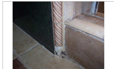
missing trim tile at shower stem wall. Recommend patching for water tightness
