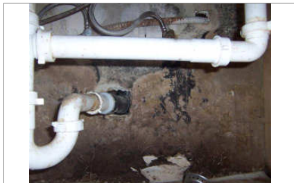
excessive mold like substance below sink.....
