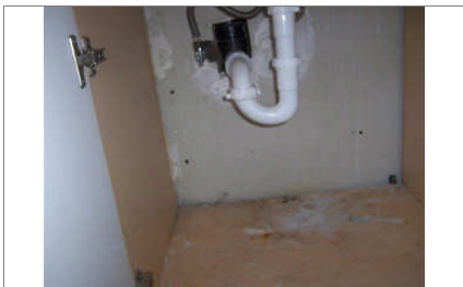
moisture stains under various bathroom sinks
