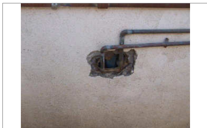
various openings around plumbing penetrations need repair/sealed
