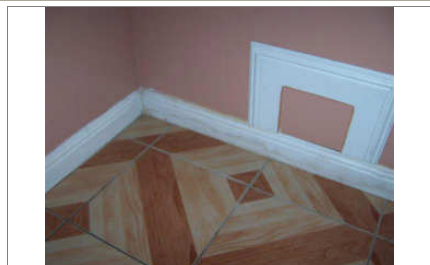
possible previous leak
