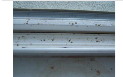
showing signs of minor mold spore buildup
